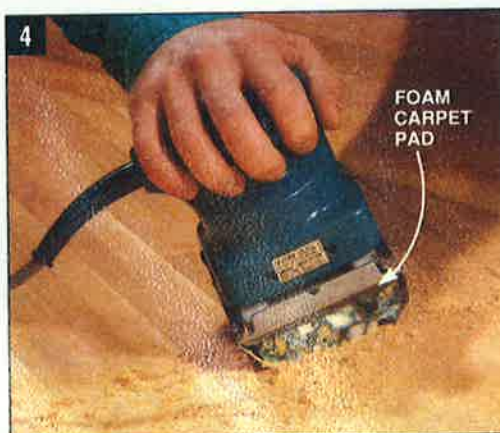
4 SAND THE INSIDE using an orbital sander. Place carpet pad between the sander's pad and the sandpaper so it conforms to the canoe's shape.
